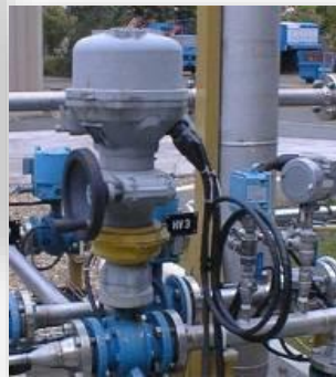
Gas shut-off valve
