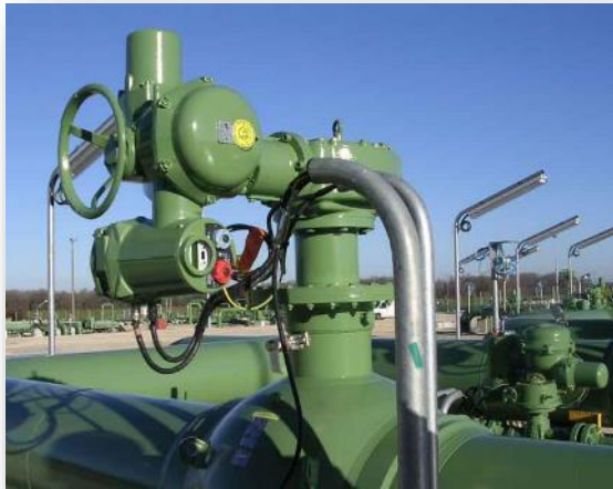
Pipeline flow control
