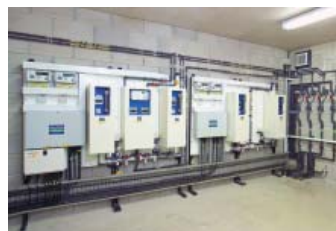
Duty/Standby Chlorine Gas Feeder Systems
