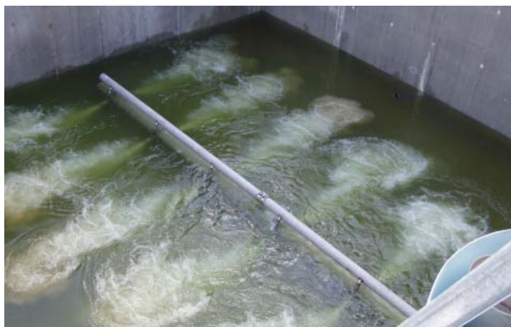
Severn Trent Services Jet Aeration Sequencing Batch Reactors
